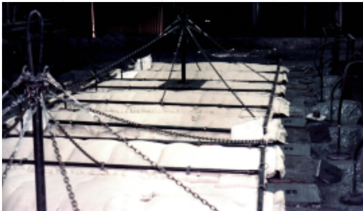
Pit Cover Blankets and Frame covering one full section on open top furnace.
